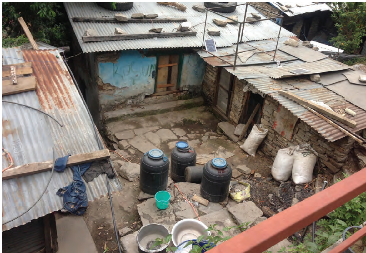
Damaged houses still in use at Kartike Bazaar. Photo by Bina Limbu
