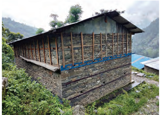
A non-compliant stone house with correction measure of wooden grids applied to support the gable wall. Photo by Manoj Suji
