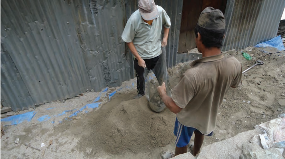
Two men sifting sand to build a house at Kartike; one man (on the right) is the house-owner and another man (on the left) is a waged labourer. Photo by Manoj Suji
