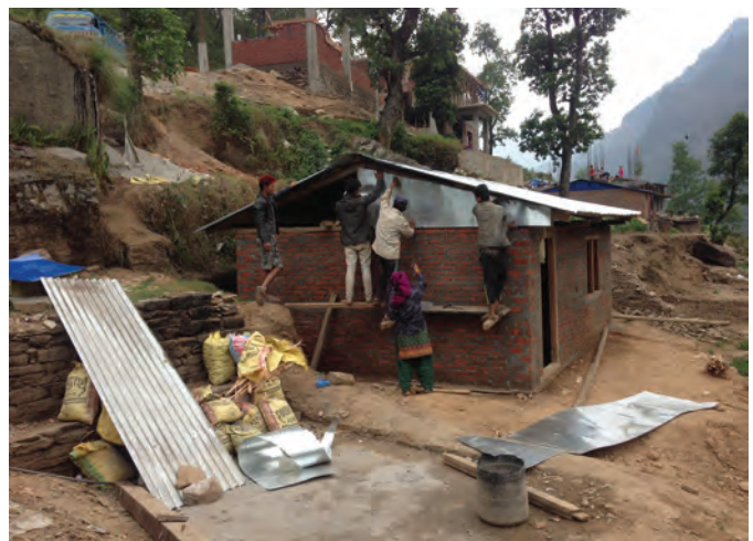
A brick-masonry house being constructed above Kartike Bazaar. Photo by Prakash Chandra Subedi
