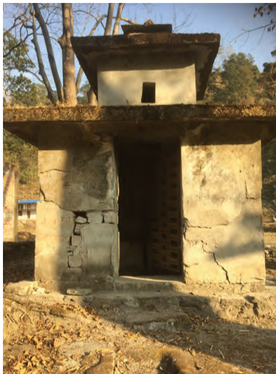
A shiva temple damaged by the 2015 earthquakes at Manje. Photo by Bina Limbu
