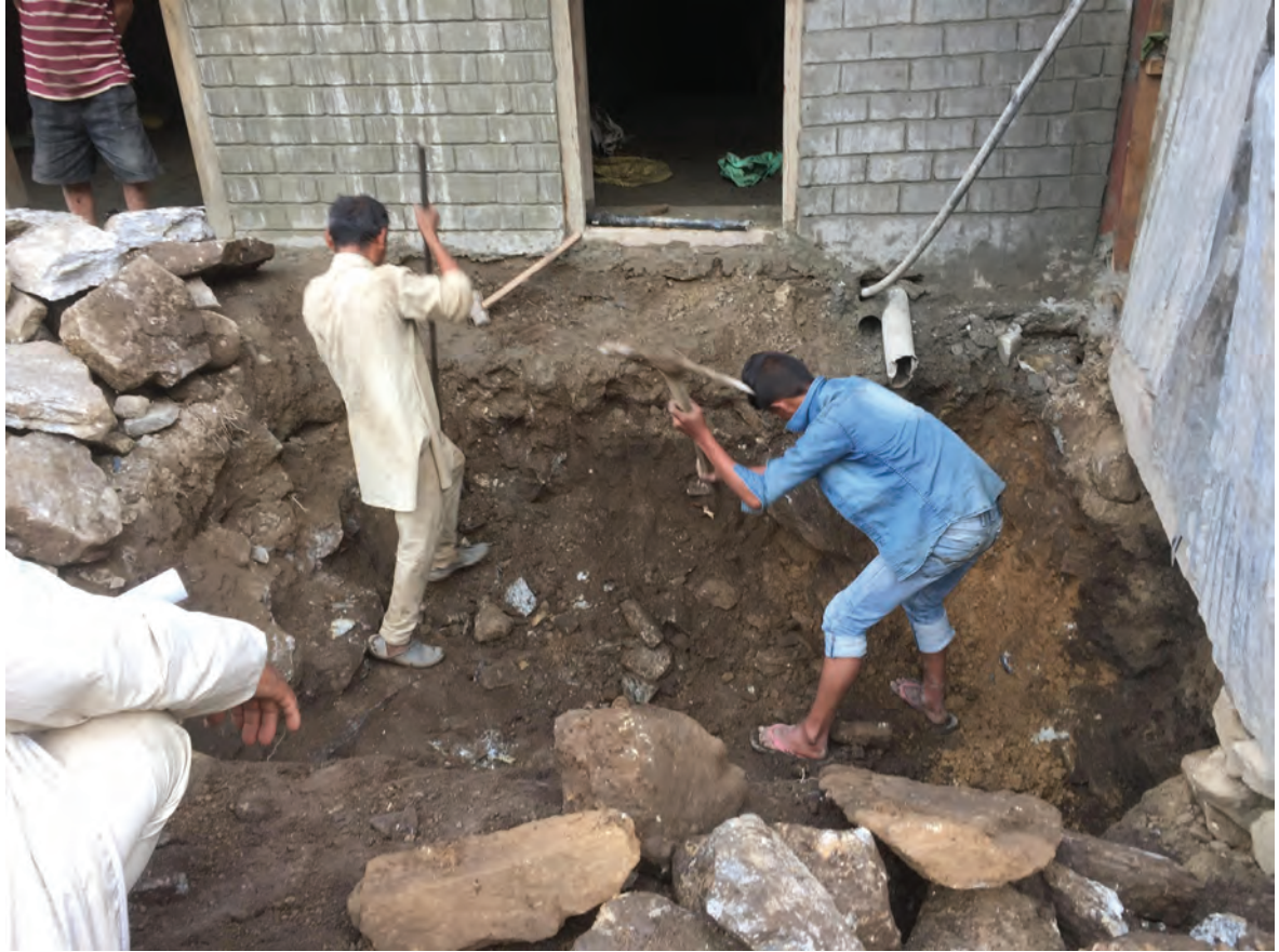
Labourers building a toilet septic tank for a house at Manje. Photo by Bina Limbu
